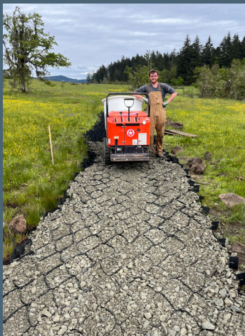
Trails Intern, Jalen McNulty, installs geocell and gravel to allow improved subsurface water flow through east Trail 3.
